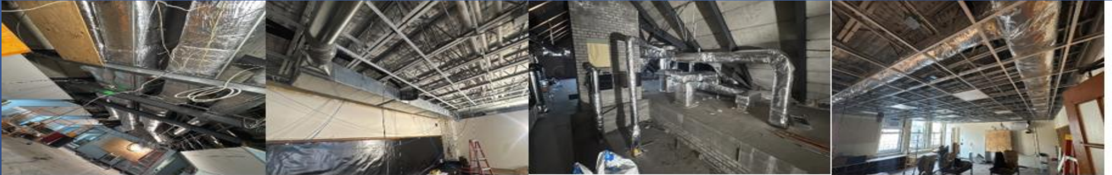
New Dedicated Outdoor Air System Ductwork
