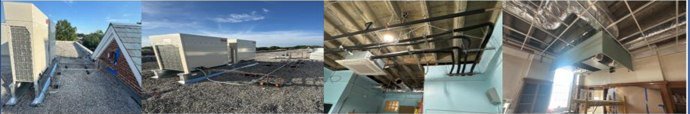
New HVAC Equipment
