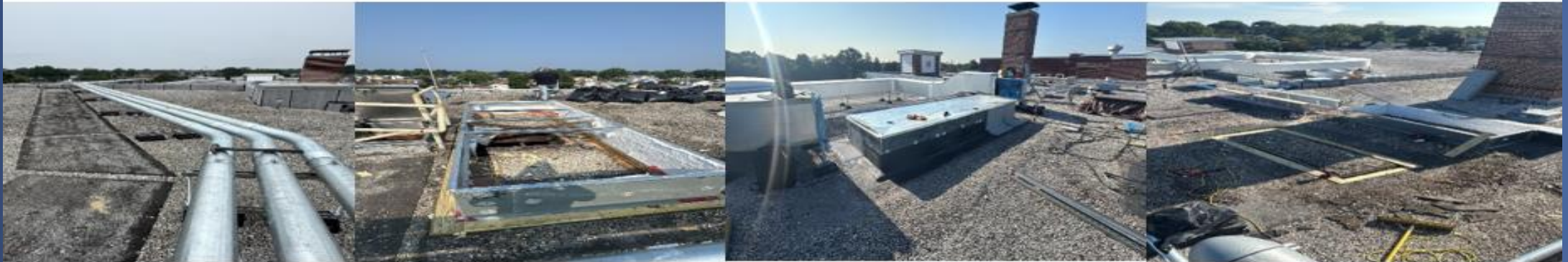
ROOFTOP ELECTRICAL PIPING AND ROOF CURBS FOR NEW HVAC SYSTEMS
